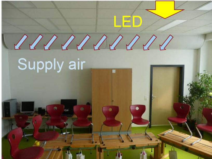
Supply Air in Classroom
