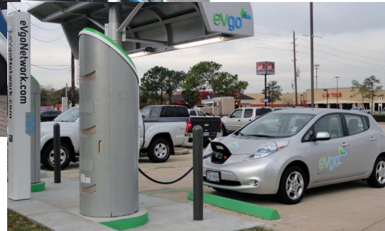
> 50 kW DC Fast Charging
