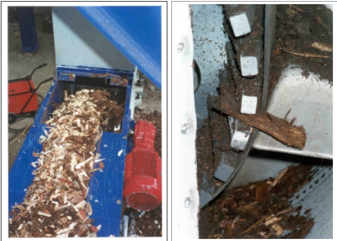
Photo 2: Problems at the Vertical Belt Conveyor
