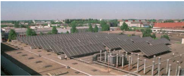
Figure 27: A 2400 m 2 collector array for an industrial application in the food industry.
