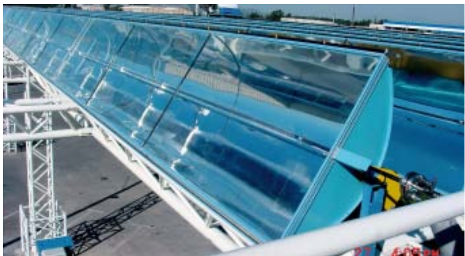
Fig. 17: 860 m 2 of small parabolic trough collectors installed at SOLEL headquarters in Beith Shemesh, Israel (picture source: SOLEL, Israel)
