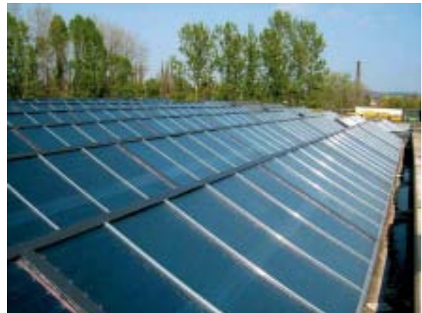
Solar plant 'AEVG Graz'
