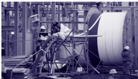
A recent demonstration project of new HTS cable design enabling large amounts of power transmission through unusually small ducts.
