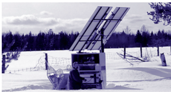
A PV hybrid (PV/propane generator/battery storage) provides electricity to a remote residence (Canada).
