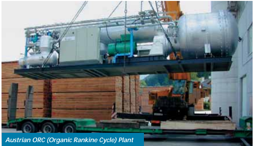
Austrian ORC (Organic Rankine Cycle) Plant New ORC plant (rated power 400 kW e ), which started operation in 1999 within the scope of a demonstration project in the STIA wood processing company at Admont, Austria; it features comprehensive technical improvements in the field of decentralized biomass combined heat and power plants.
