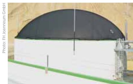
Biogas facility St. Veit / Glan
