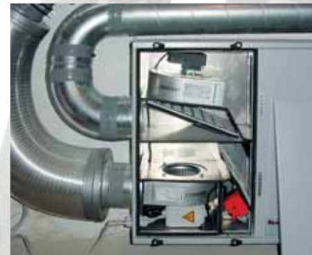
Blower unit of a ventilation appliance.
