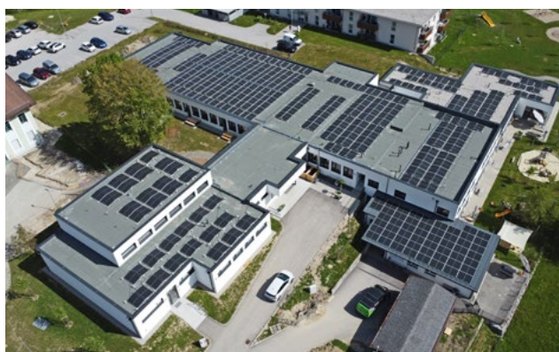
230 kWp PV system, Neukirchen primary and nursery school, photo: Alexander Strobl
