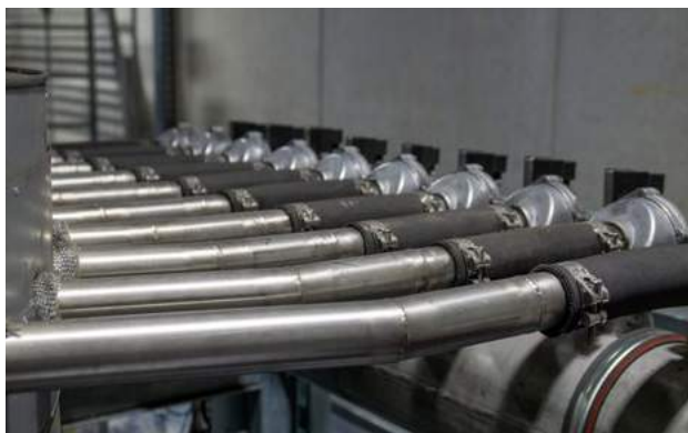
Wood gas CHP plant: Wood gas processing via hot gas filtration, photo: BEST / Lagler
