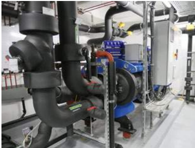
From left: server room as heat source, heat exchanger between server racks, pressure equalizer, chiller. Photos: Waldhör KG
