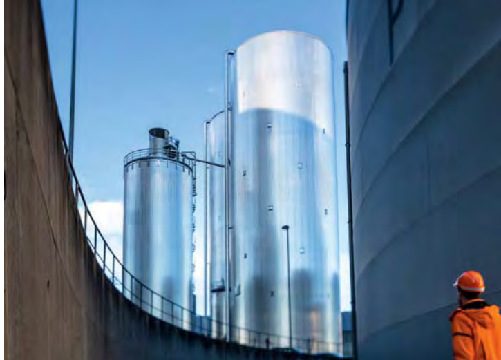
Heat storage facility, source: Wien Energie/Ian Ehm
