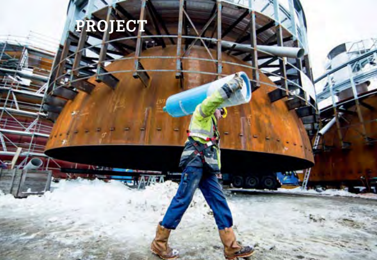
Construction of the high-pressure heat storage facility in progress, source: Wien Energie/Ian Ehm
