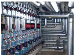
Nerve centre of a large heating system, Source: Ashkan Nasirkhani, fotolia.de
