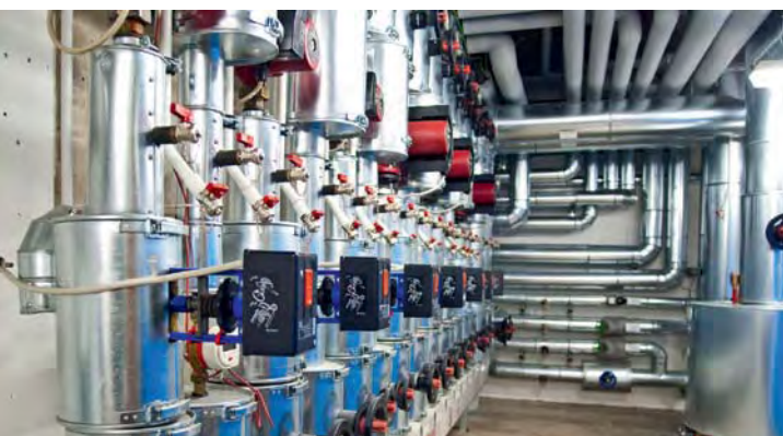
District Heating Network - Building connection. Source: Ashkan Nasirkhani, fotolia.de
