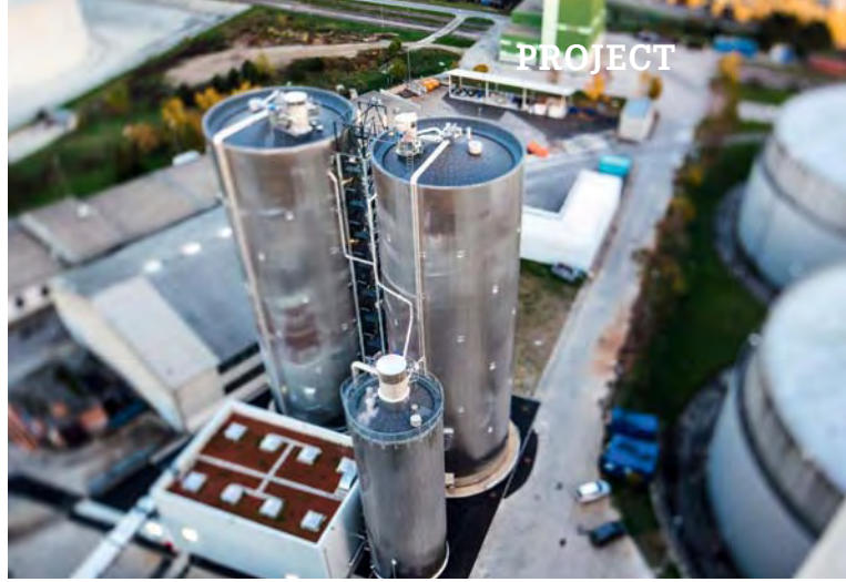
High-pressure heat storage facility at Simmering power station, source: Wien Energie/Ian Ehm
