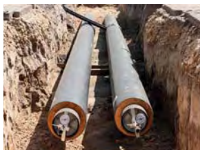
District heating lines, Source: fefufoto, fotolia.de
