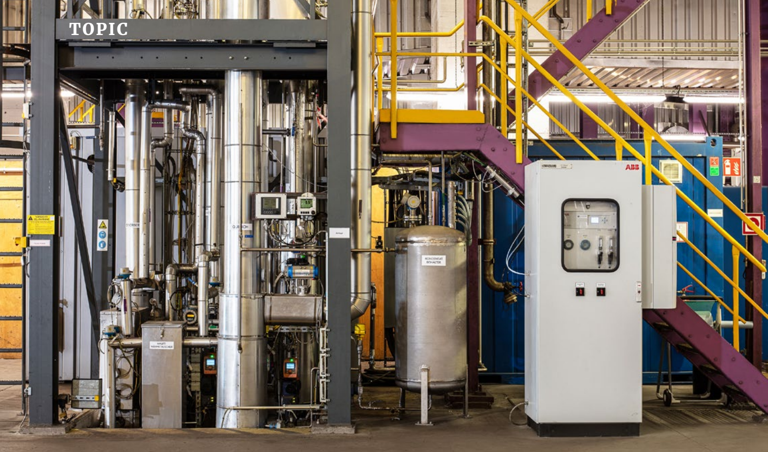
Amine scrubber for capturing CO 2 photo: voestalpine Stahl GmbH
