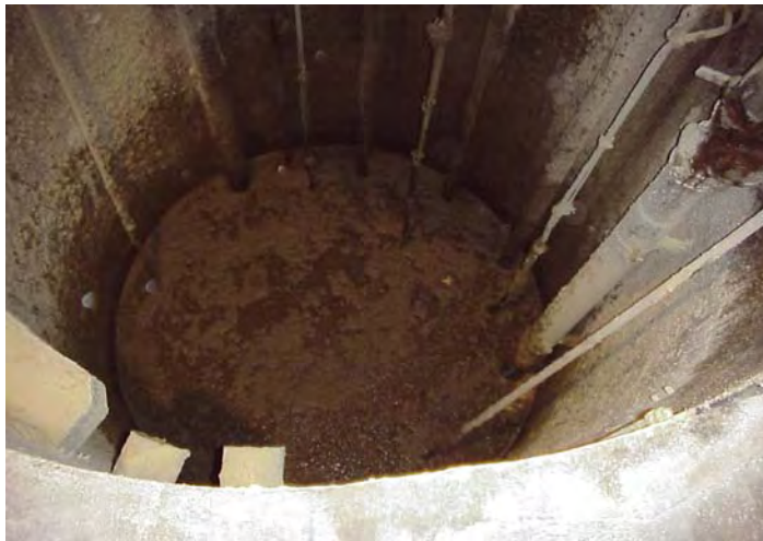
Photograph 6.4: View into the underground mixing tank of the biogas plant Paldau
