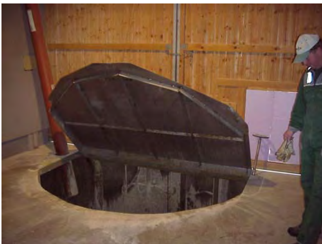
Photograph 6.3: Underground mixing tank of Biogas plant Paldau
