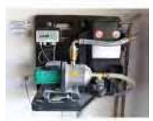
↑ Illustration 353 : Pump installation
