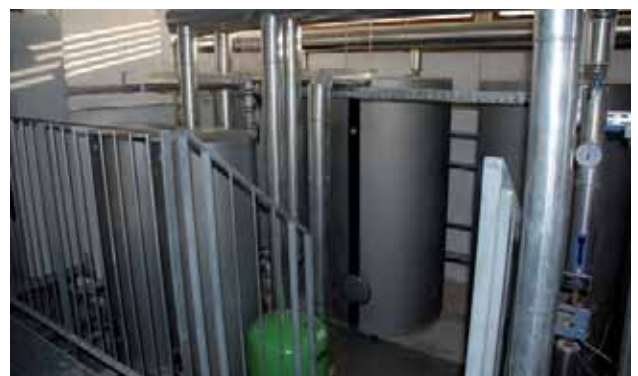
↑ Illustration 250 : Insulation of the distribution network
