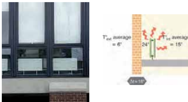
↑ Illustration 235 : Radiators in front of a non insulated wall (glazed or not).
