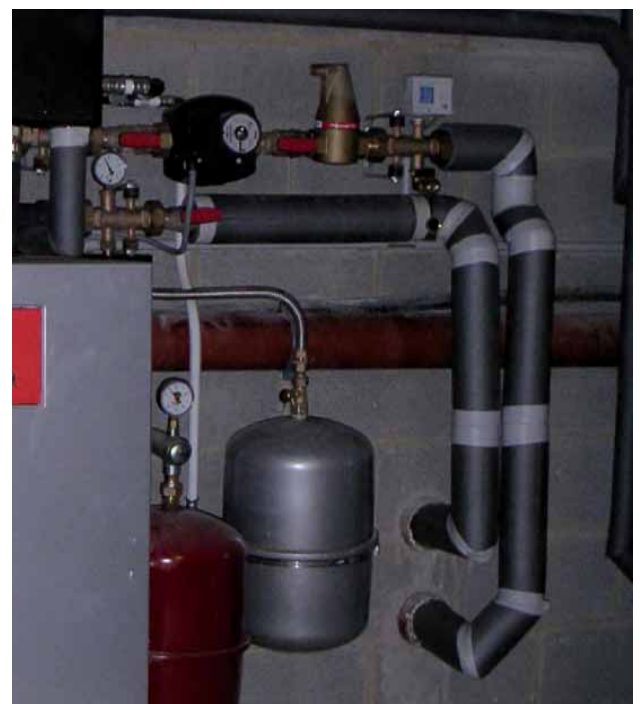
↑ Illustration 233 : Insulation of the distribution network.
