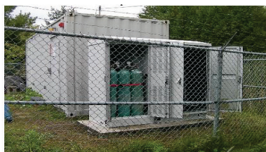
Example of an outdoor cabinet for fuel cell and outdoor fuel storage (10 kW / 90 kWh solution) - next to a shelter.
