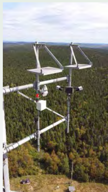
Figure 2. Ice detectors and fog sensors (credit: NRCan)
