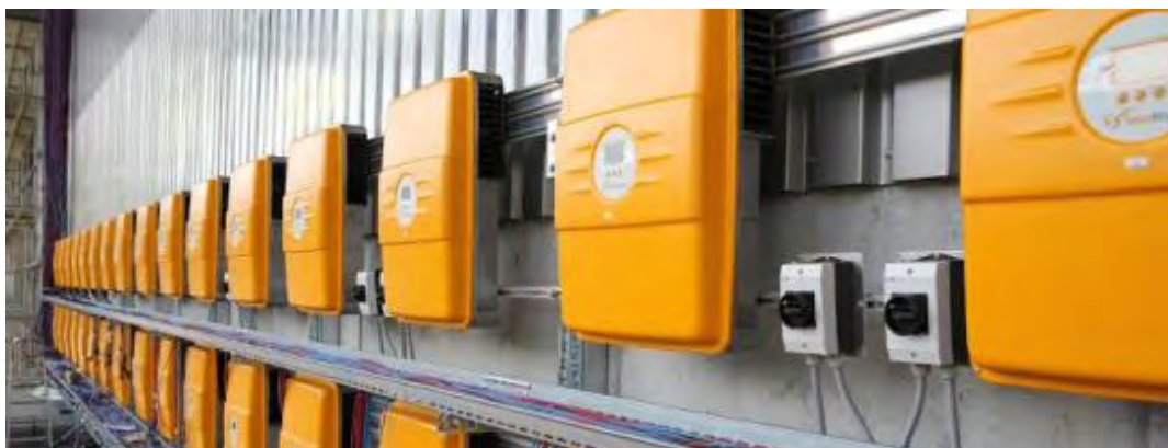
Inverters at a 555 kW commercial PV plant, Kölliken, Switzerland – Courtesy of EcoenergieA+, Schöftland, Switzerland
