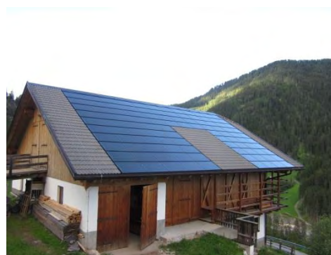
BIPV systems with monocrystalline cells, 20 kW, Bolzano, Italy, courtesy of GSE
