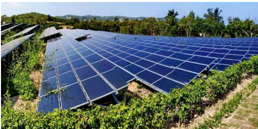
600 kW PV, Dongao Island, Guangdong, China, Courtesy of Lu Fang
