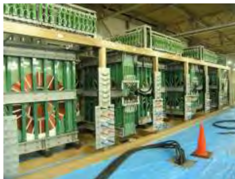
Figure 4.7.5-9: 66kV transmission line emulator
