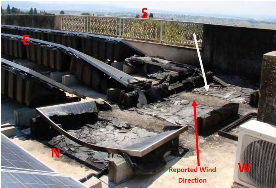
Figure 34: Fire due to junction box connection problems.
