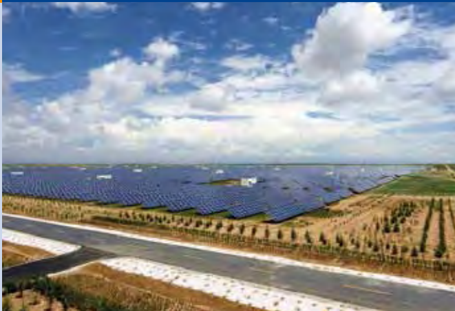
Fig. 3 – 520 MW Longyangxia Hydropower PV station, Gonghe, Qinghai, China (Photo: Yellow River Hydropower Company).
