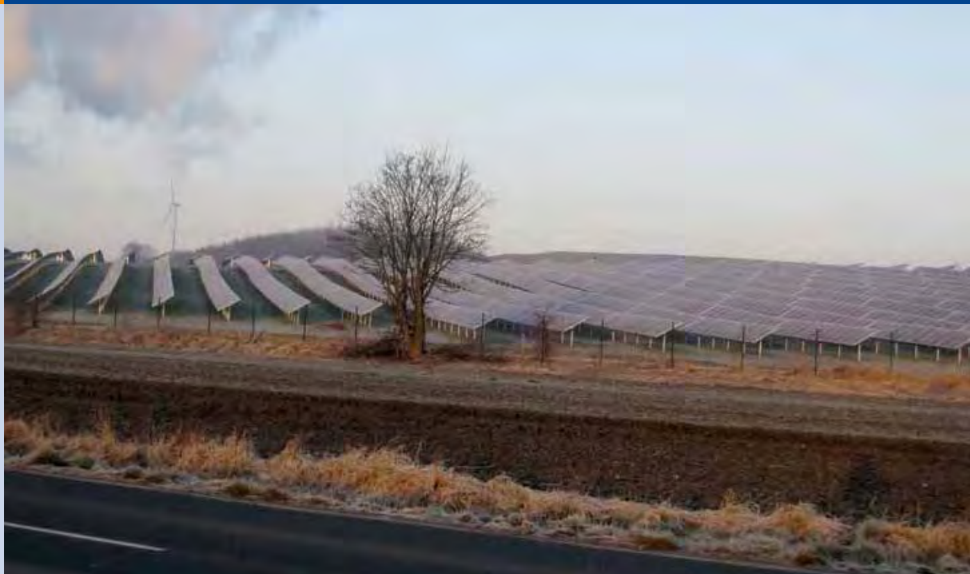
Fig. 2 - Ground mounted photovoltaic installation with 3,9 MW peak power on a former landfill site (Photo: Klaus Prume).
