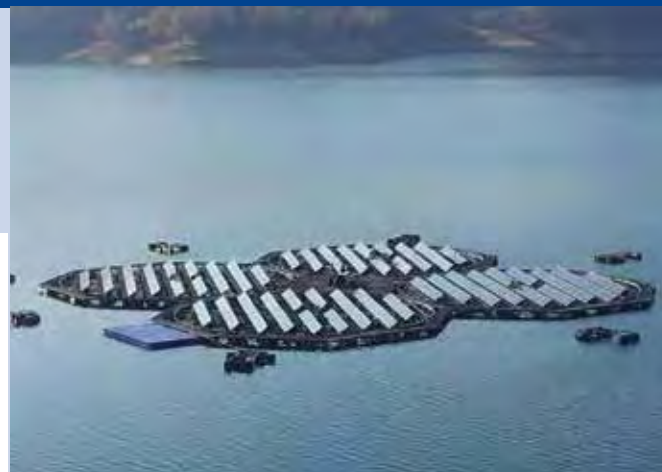
Fig. 3 - 100 kW tracking-type PV power plant on the water surface at Hapcheon Dam, Hapcheon-gun, Gyeongsangnam-do, Korea.
