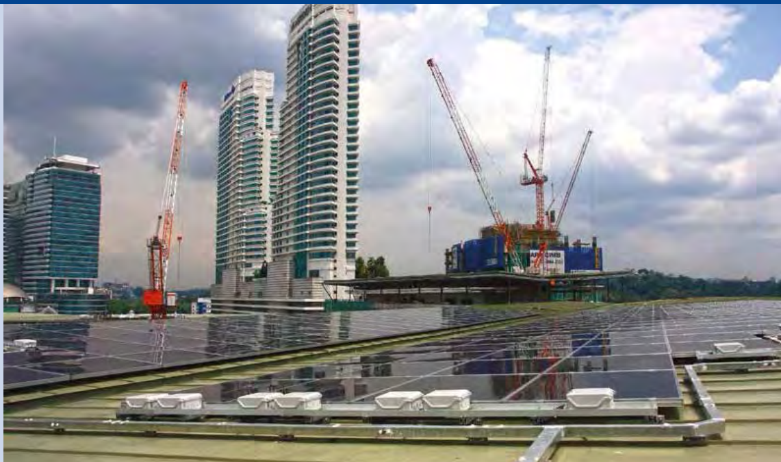
Fig. 1 - Lot E, KL Sentral (168kWp), Platinum rated "Green Building" (Photo: Pekat Teknologi Sdn Bhd).
