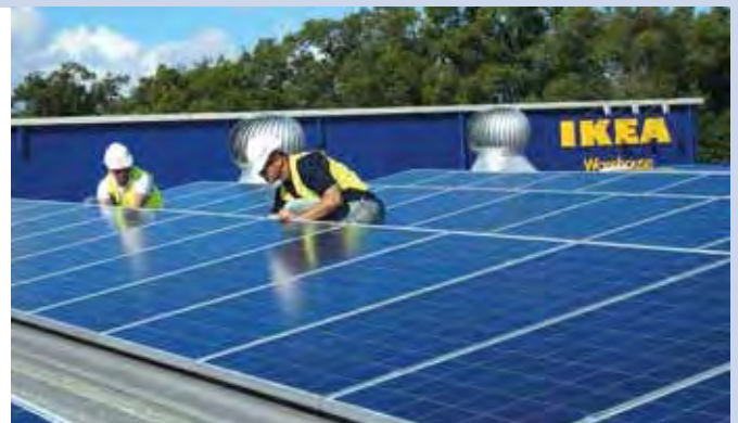
Fig. 2 – IKEA's 3,6 MW Commercial PV Roll-out in Rhodes, NSW (Photo: Canadian Solar, Australia).
