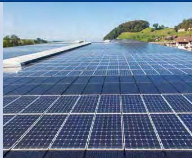
Fig. 3 - 538 kW roof-integrated PV system, Affentranger Bau AG, Altbüren (Photo: © NET Ltd. /DanielForster.com).
