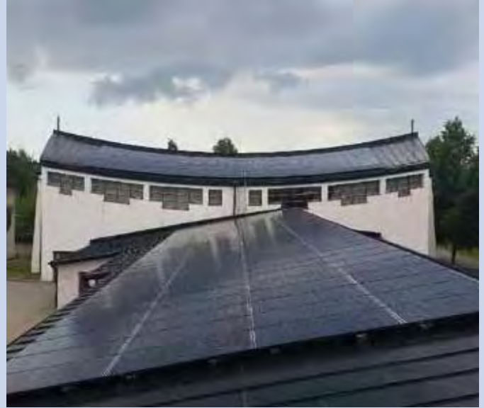
Fig. 2 - 50 kWp on a church roof. Lambohovskyrkan, Linköping (Photo: PPAM.se Sweden AB).
