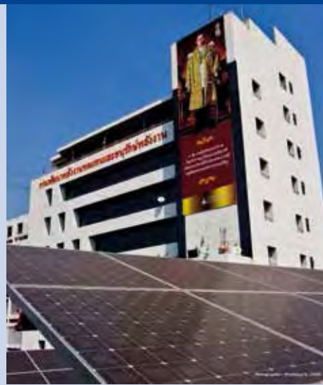
Fig. 3 - Solar PV Rooftop System 5 kWp at Department of Alternative Energy Development and Efficiency, Bangkok, Thailand.
