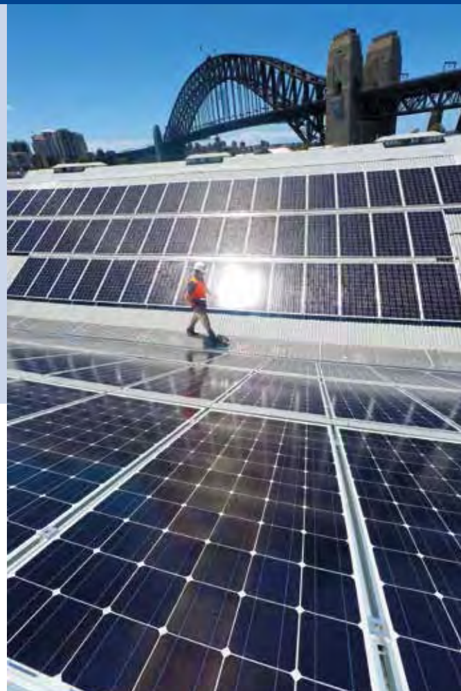
Fig. 4 - Sydney Theatre Company rooftop system (Photo: SF-Suntech).
