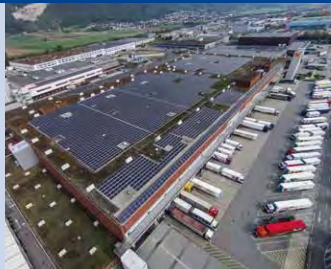
Fig. 7 - 32 000 m 2 PV system with 5,2 MWp, producing 6,8 GWh per year, Migros, Neuendorf (Photo: © NET Ltd. /DanielForster.com).
