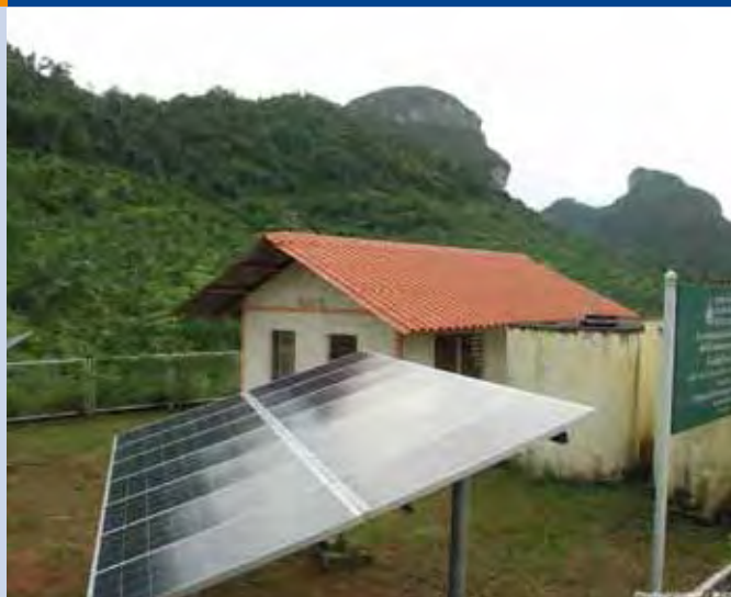
Fig. 2 - Solar PV Off-Grid System 2 kWp at Koh Phaluai School by Department of Alternative Energy Development and Efficiency, at Phaluai Island (Green Island), Suratthani, Thailand.
