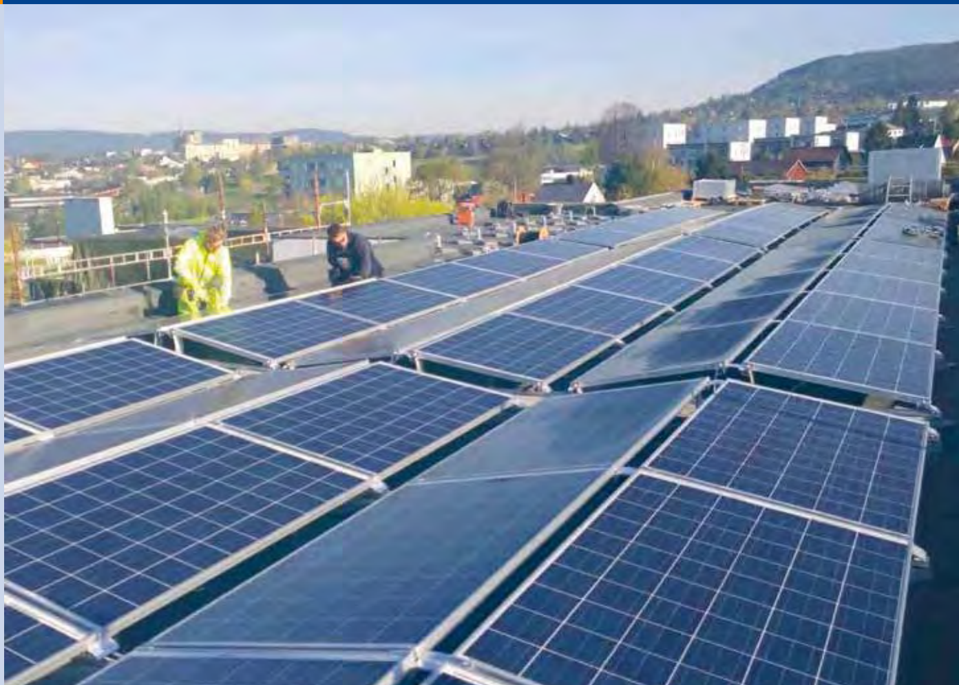
Fig. 2 - Omsorgsbygg Oslo installed a 130 kWp system at Økern Sykehjem (a home for elderly people). The power from the system is for self-consumption (Photo: Fusen AS).
