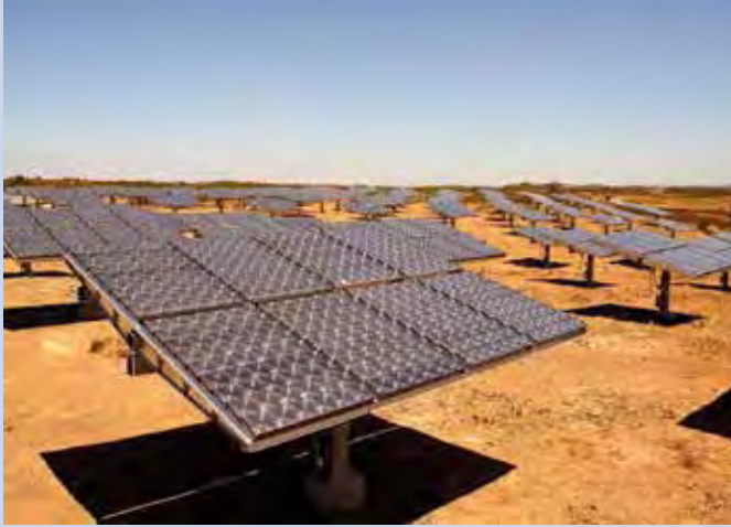
Fig. 1 - Capwatt - Martim Longo HCPV Plant - 2 MW (photo: Pedro Lobo).
