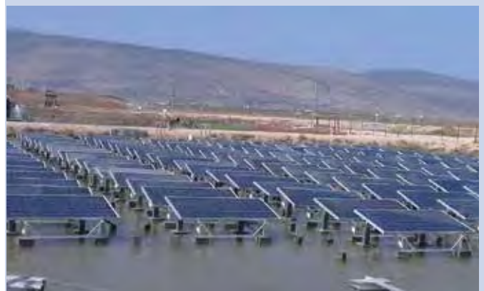
Fig. 3 - Solaris Synergy's solar PV field installation on a water reservoir.
