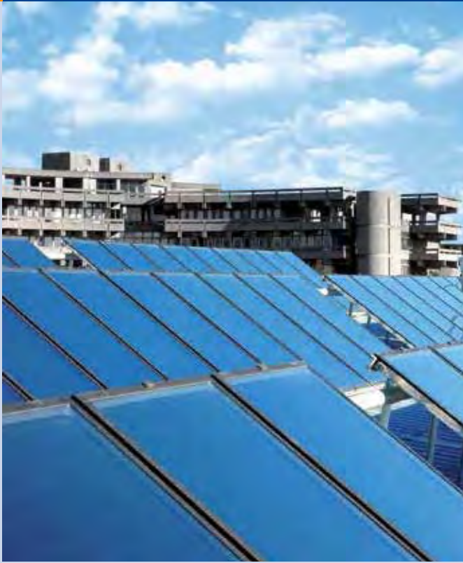
Fig. 2 - Roof top solar panels medium sized system, the Netherlands.
