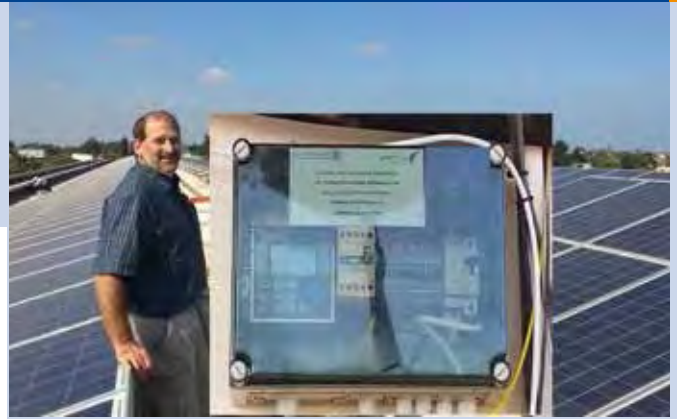
Fig. 1 - MG Lightning monitoring system at a solar PV installation.
