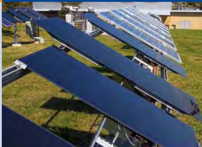
Fig. 3 - PV Outdoor Research Facility at the CSIRO Energy Centre in Newcastle Australia.
