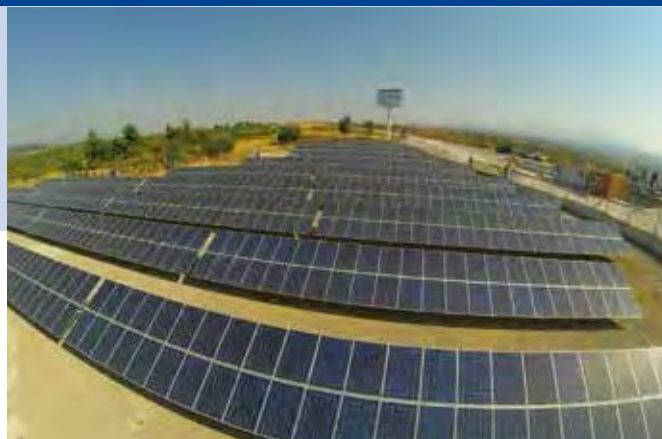
Fig. 2 - 500 kW PV system in Izmir, Turkey; one of the supported projects by IZKA.
