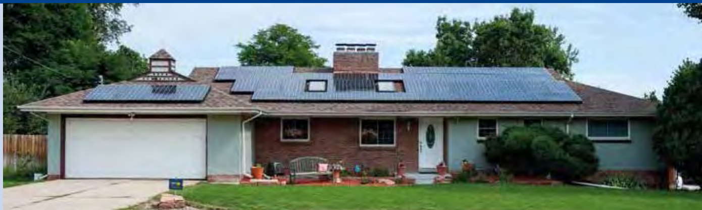
Fig. 1 - A residential home retrofitted with photovoltaic (PV) panels in Lakewood, CO (Photo: Dennis Schroeder / NREL).
