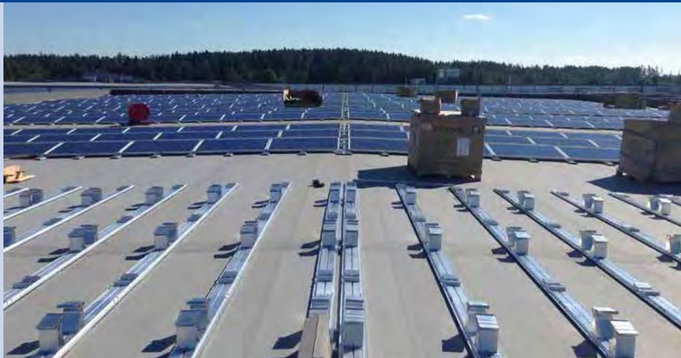
Fig. 1 - At Asko Vestby, a 370 kWp system was installed during the summer of 2014. This is the largest system in Norway, and the system is built solely for self-consumption. The power is delivered to a refrigerated storage (Photo: Multiconsult).
