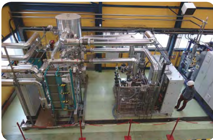
A heat pump with an output temperature up to 140 °C, with water as its working fluid.
