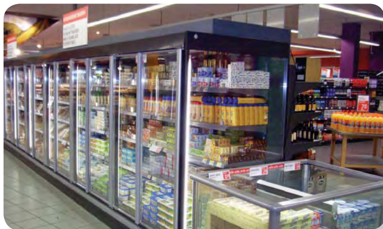
Supermarket refrigeration installation.
