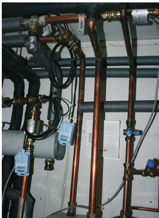
Heat pump installation, not a good example
