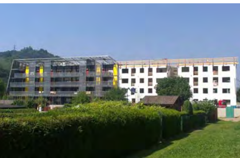
Kapfenberg case study – View of the finished renovation (left part of building) and still in renovation (right part of building). Source: AEE – Institute for Sustainable Technologies
