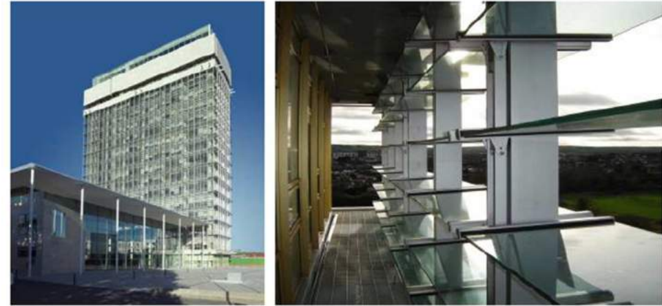
Figure 1: External View of the refurbished building (left) and detail of retrofitted second skin with automated glazed louvres (right)
