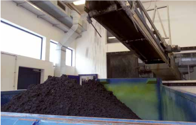
Figure 5: Dewatered sewage sludge
