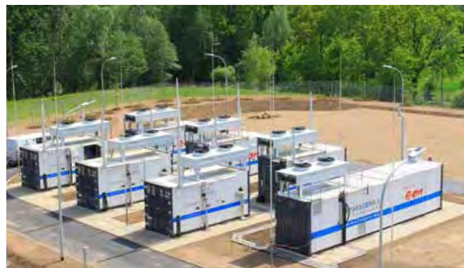
Figure 9: 2MW Power to gas unit based on alkaline electrolysis in Falkenhagen, Germany. The hydrogen is injected into the gas grid without methanation. (Source: E.ON)
