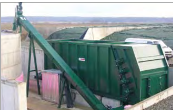
Photo 7: Silage dosing unit (back) with spiral elevator (front). The silage clamps can be seen in the back.
