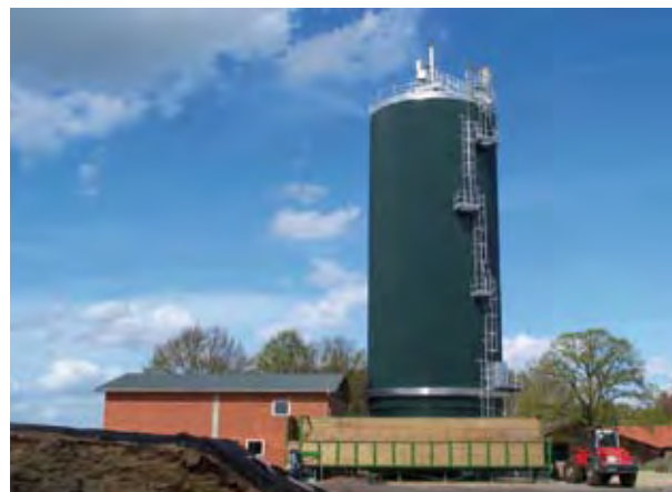
Photo 15: Dry continuous digestion
