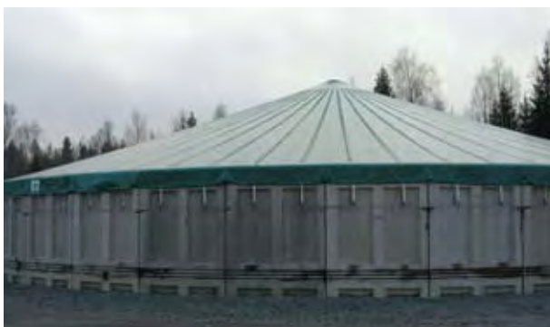
Photo 9: Gas tight coverage of a post storage tank for digestate in Sweden. Residual biogas developed from digestate is collected for energy use, while greenhouse gas and ammonia emissions are prevented.
