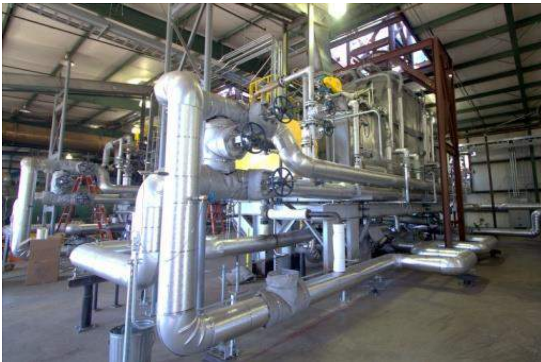
Figure 4-5 The torrefaction reactor of Solvay Biomass Energy
