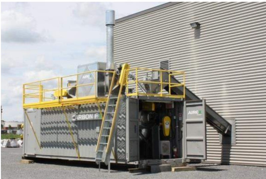
Figure 4-8 Cyclonic reactor and combustor of the Airex installation.
