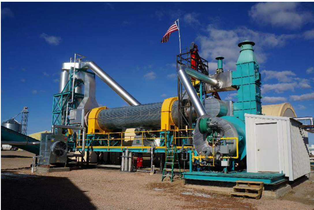
Figure 4-7 Rotary drum torrefaction island delivered by TSI.
