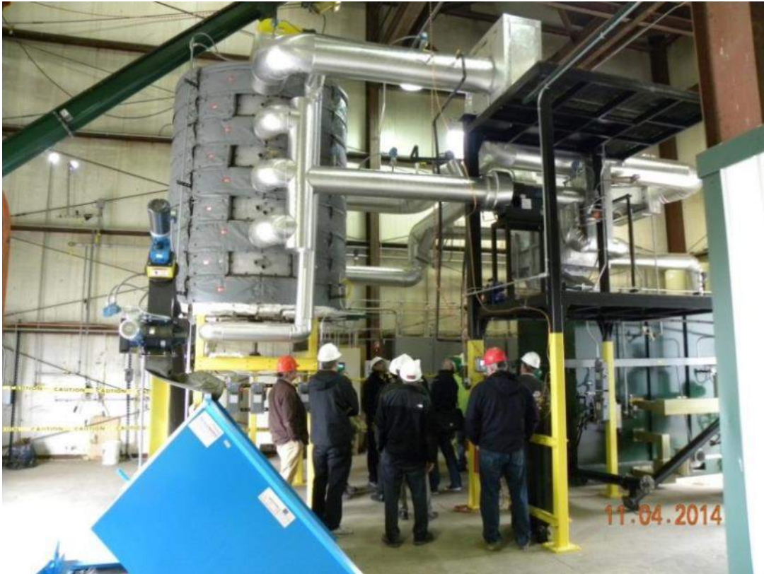
Figure 4-14 TGE Torrefaction Reactor System.
