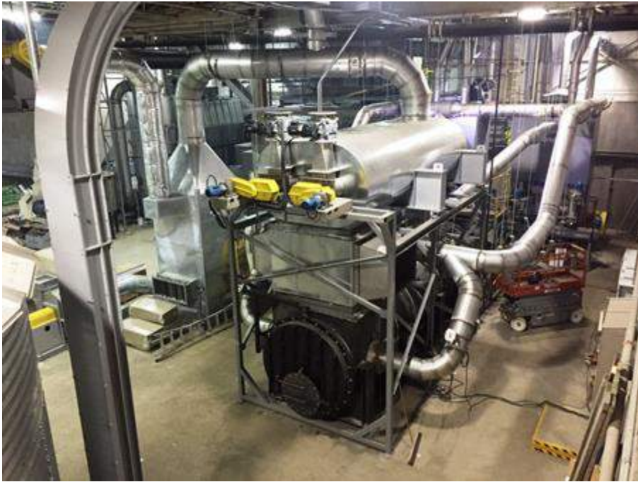
Figure 4-9 Airex demonstration plant, Becancour.
