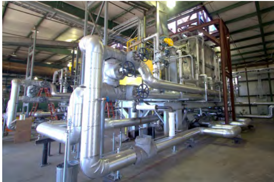
Figure 7.7 The NBE torrefaction Reactor
