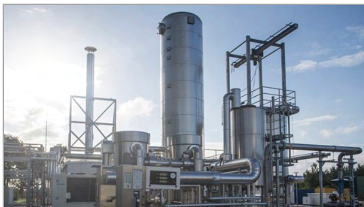
Fig. 2 Power-to-gas Plant to Produce E-gas (Source: Audi AG)
