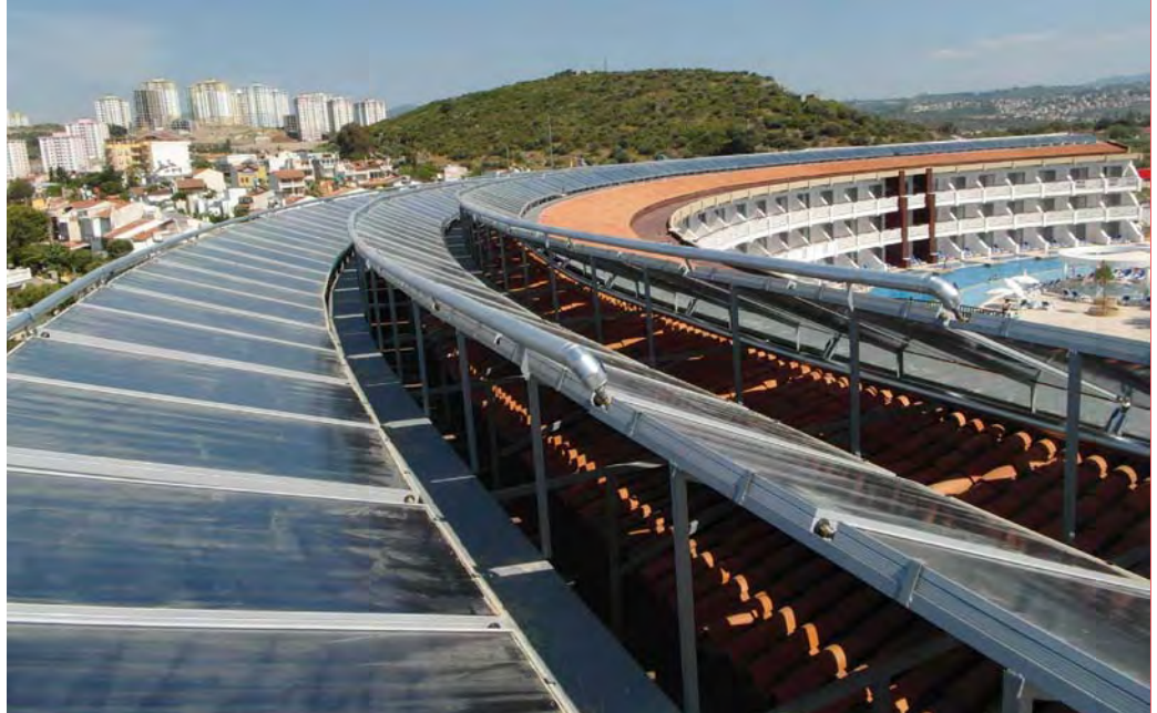
▲ Solar thermal application for hot water production at the Ephesia Hotel in Kusadasi on the Aegean coast.
