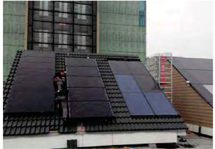
▲ BIPV project SolarBeat. Left PVT panels, middle PV panels and right 3 PVT panels and 3 solar thermal collectors.
