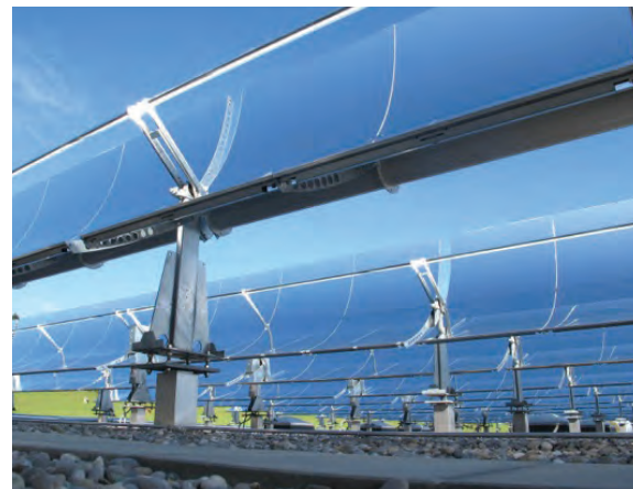
▲ On Sun: NEP Solar collector field on the rooftop of the Tête de Moine cheese factory in Saignelégier, Switzerland.
