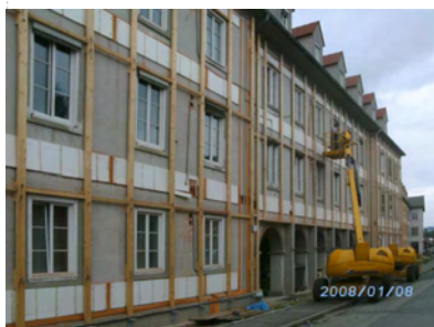
Figure 16: Heat dissipation on the outside of the existing walls.
