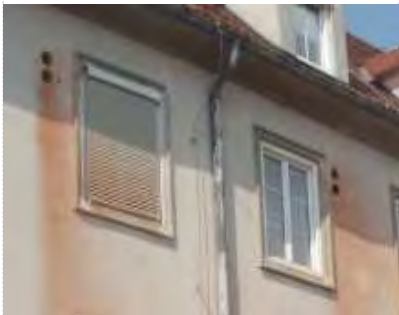
Figure 11: Boreholes in the existing wall – no penetration before completion
