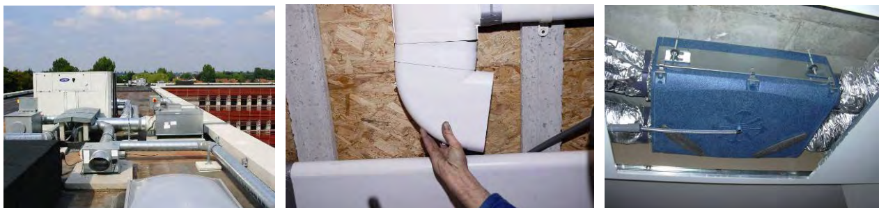
Figure 27: Installing fan/extractor units on flat roof, installing ventilation ducts, installing heat exchangers
