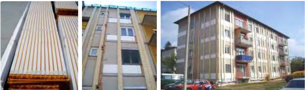
Figure 24: Heat dissipation system installed on the outside of the exterior wall (Source: AEE INTEC)
