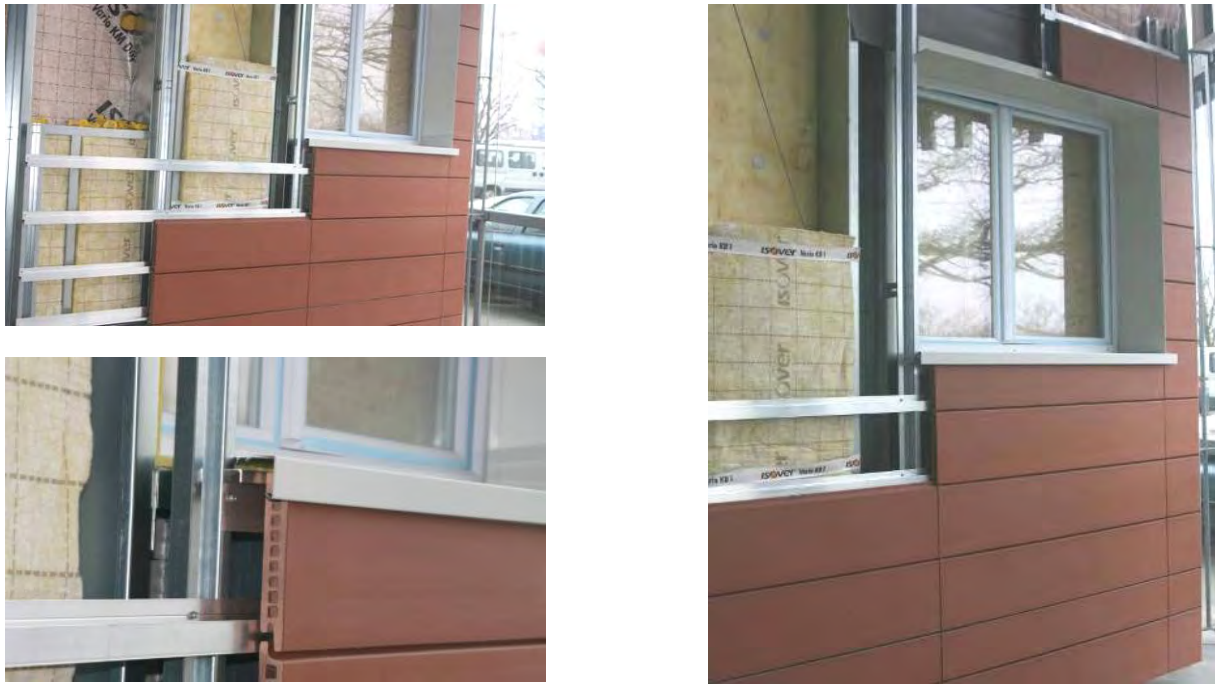
Figure 21: Mounting of cladding (ATLAS facing by VETISOL)
