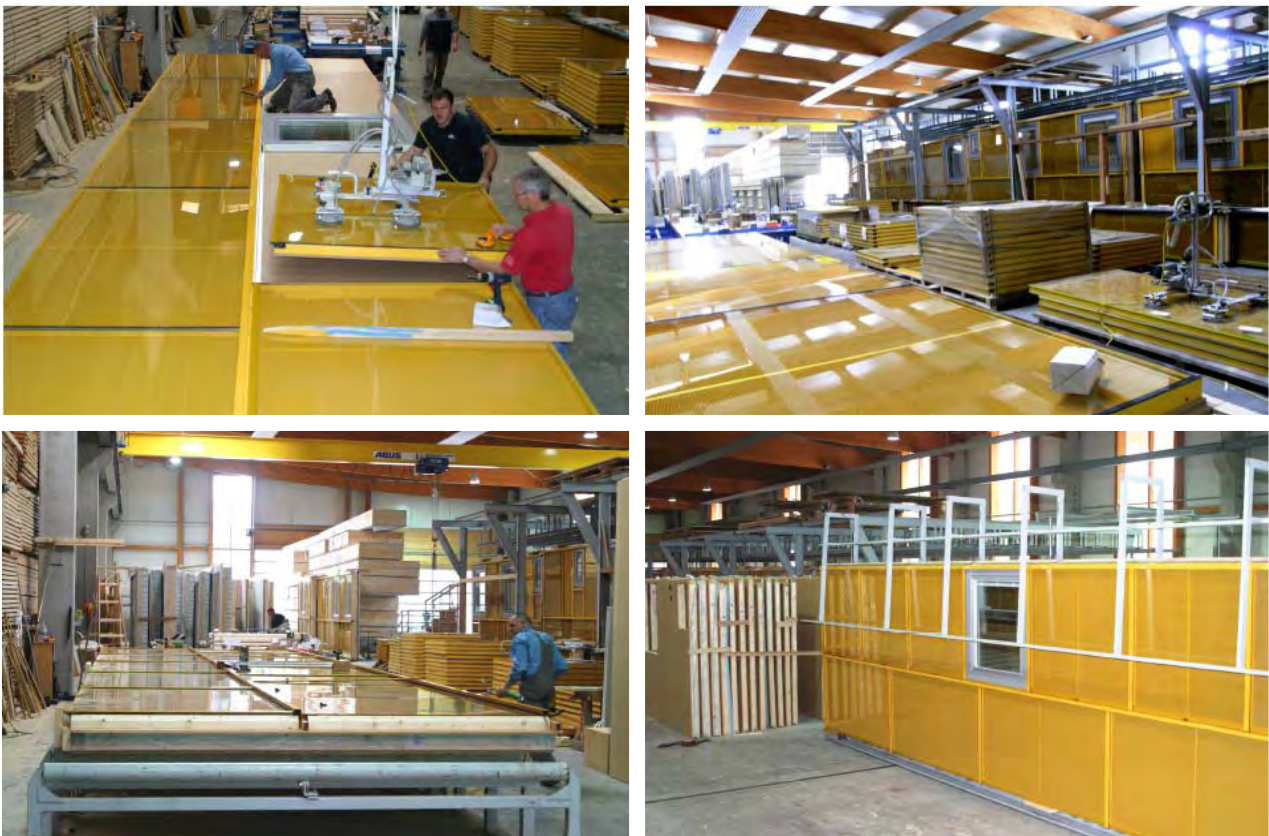
Figure 16: Assembling procedure in the fabrication of the carpentry Kulmer Bau (Source: gap-solution GmbH)
