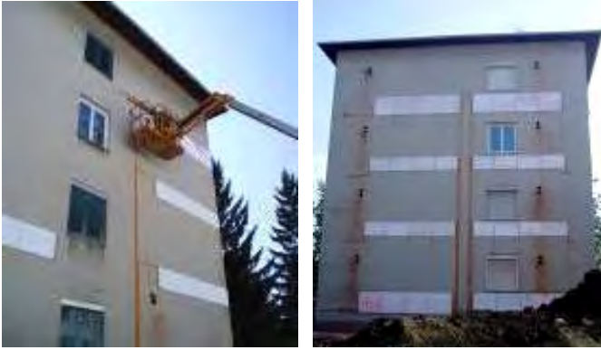
Figure 23: Two views on the exterior walls during installation works. The heat dissipation (XPS-boards with inserted heating pipes) is assembled in the wall-areas below the windows (Source: AEE INTEC)
