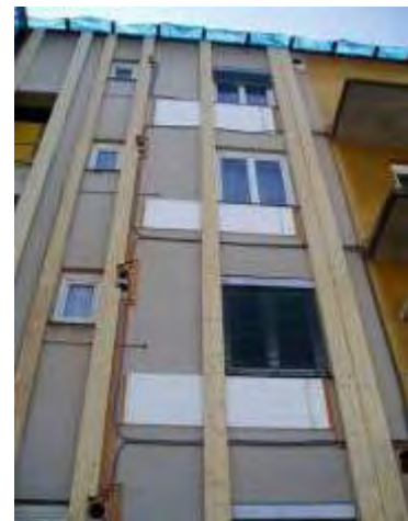
Figure 13: Photo during renovation works on the exterior wall with the levelling laths assembled on and in-between the insulation panels with inserted heating pipes.
