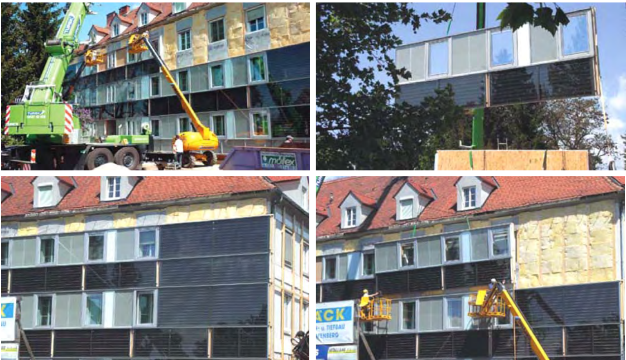
Figure 25: Assembling procedure of the façade modules with integrated collectors (Source: AEE INTEC)
