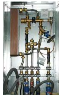
Figure 33: Transfer station installed inside a building
