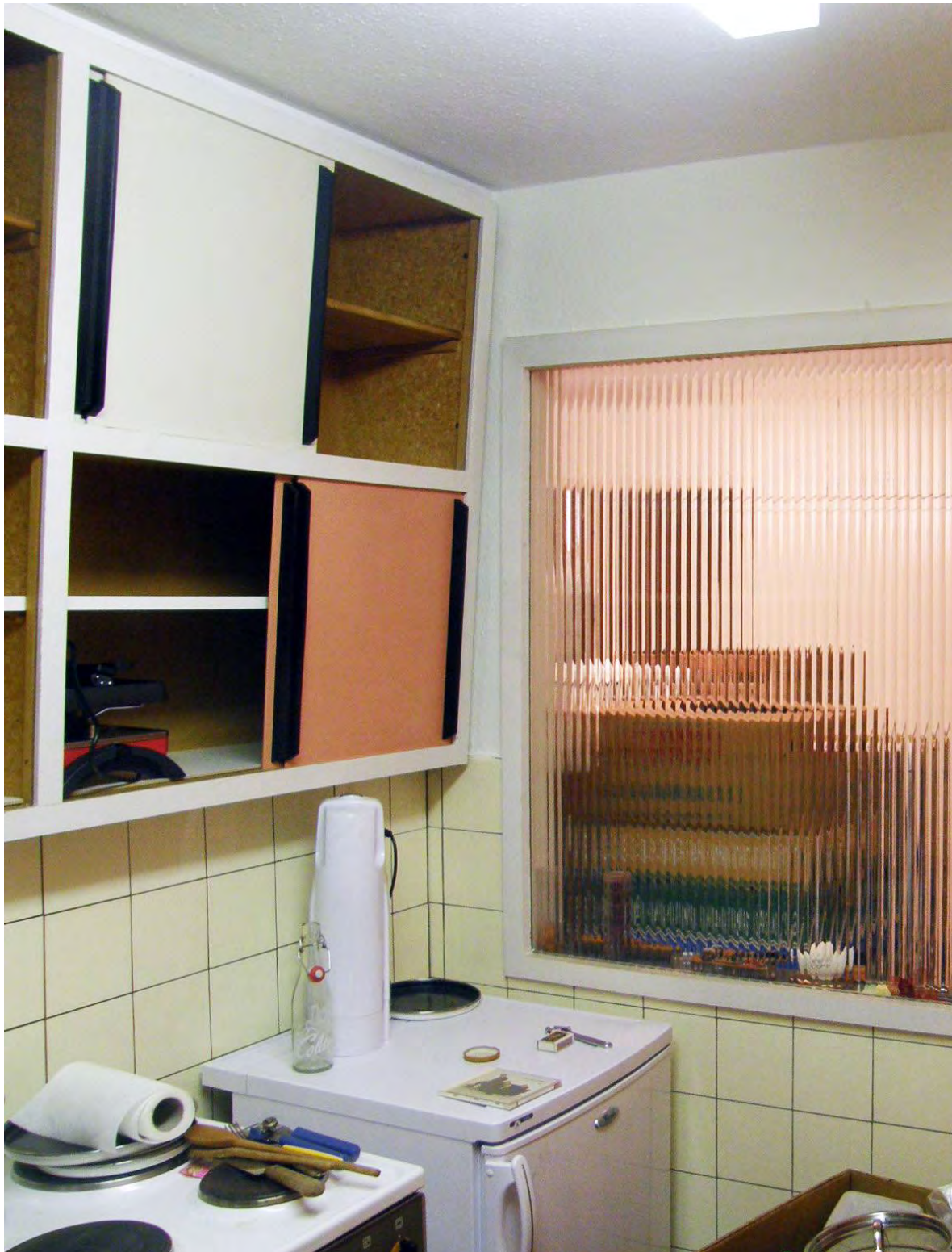
Original 1950 kitchen of case study building, Lucerne (see chapter 6.5), photo by R. Fischer, HSLU-CCTP
