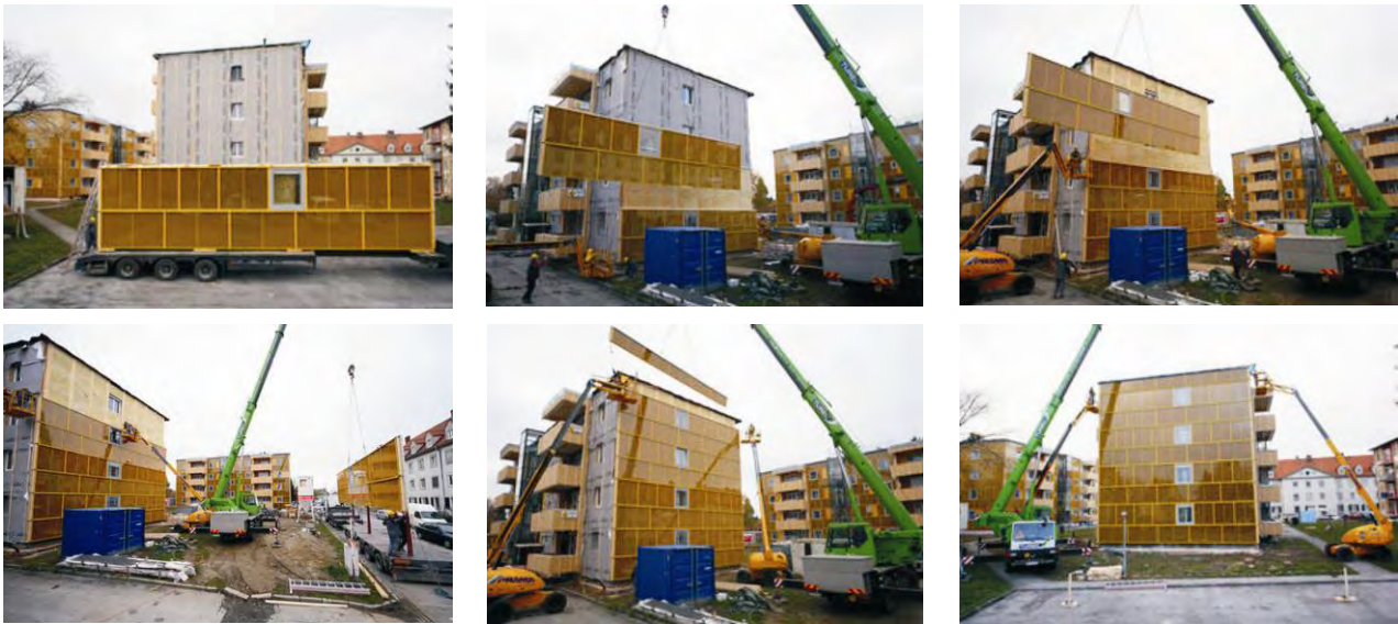
Figure 2: Assembling procedure of prefabricated façade modules within the renovation “Dieselweg”, Graz-Liebenau (Source: gap-solution)
