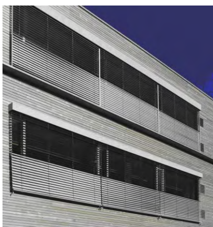
Figure 27: External venetian blinds, upper part adjustable for optimized daylight transport.
