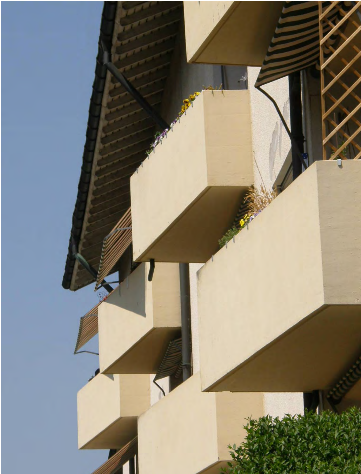
Southwest façade of case study building, Lucerne (see chapter 6.5), photo by R. Fischer, HSLU-CCTP
