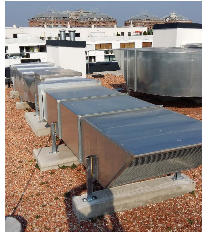
Exhaust ventilator on roof source: Peter Holzer
