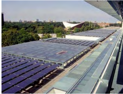
163 kWp PV system on a government building, Germany
