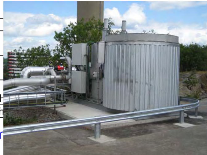
Converter after water scrubbing
