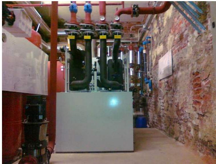
Figure 21: Heat Pump System 55
