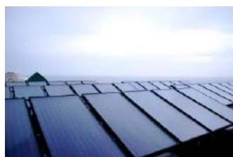
Figure 12: Large Scale Solar Plant 20
