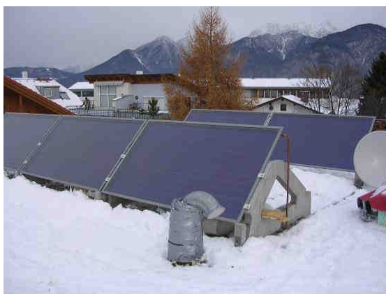
Figure 2 - collector field on the roof
