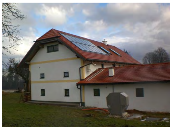
Figure 3: Single family house with heat pump unit and collector field
