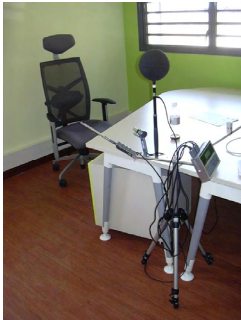
Figure 5-14 : Example of portable unit used for the spot measurements and the assessment of thermal comfort in the Enerpos Building. Indoor air temperature, indoor humidity, black globe temperature, illuminance and air velocity are measured every minute (10 seconds for air velocity) and stored every 15 minutes. Source : University of Reunion.
