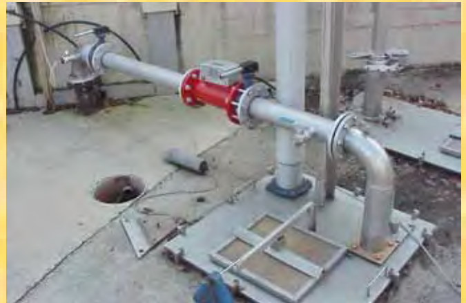
Biogas Flow Meter (Photo: P. Enzinger)
