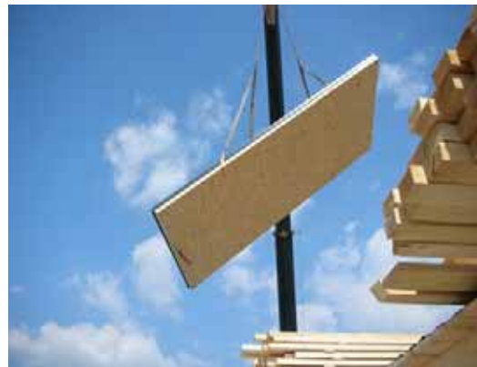
picture 29 Mounting of integrated solar collectors on the roof of an attic conversion in Graz, image source: Eduard Wasserfaller
