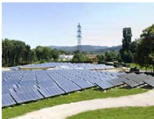
Collector area: 3855 m 2 (complete assembly in 2010) Store volume: 64.6 m 3 district heating feed-in and heating support Commissioning: 2007-2008
