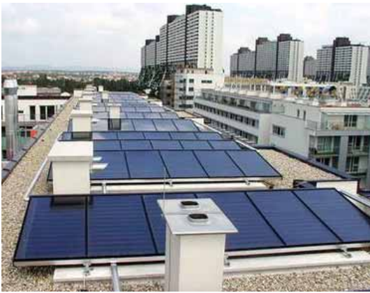
picture 27: 202 m 2 collector area on a roof of a multifamily building in Vienna (Erlaaerplatz), 200 apartments, 10 m 3 heat store, image source: S.O.L.I.D. [31]
