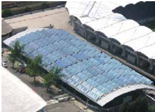
Collector area: 1407 m 2 large scale collectors application of energy: about 540 MWh/a Commissioning: 2003
