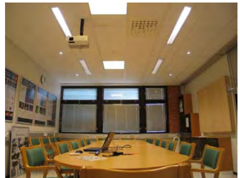
Lighting by a combination of LED and fluorescent lamps in the meeting room
