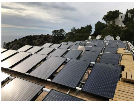
90 PVT collectors provide heat and electricity to a hotel in Spain.
