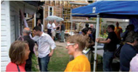
Now House mid-construction open house invites visitors to view retrofit changes prior to completion when many changes will no longer be visible.
