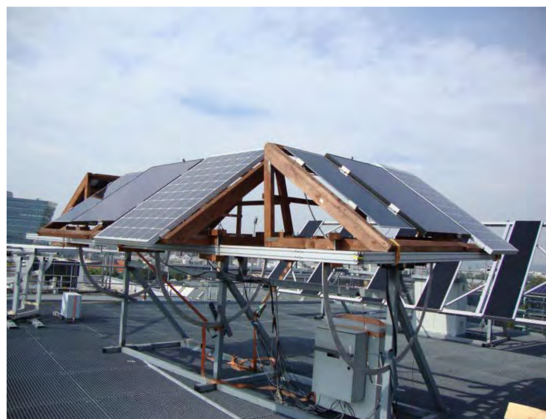
Figure 1: Outdoor test facility on the roof of AIT, Vienna. Three module types are mounted towards east west, south and west with an inclination of 35 degrees.
