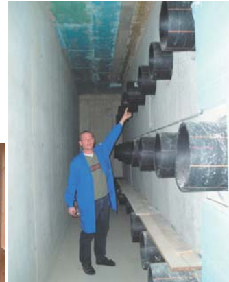
Erdkollektoren | Sub-soil collector
